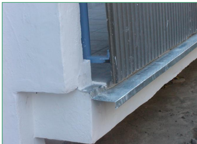
Detail lodžiovej dosky pri odkvape po obnove Detail of loggia board at the cornice following renovation
